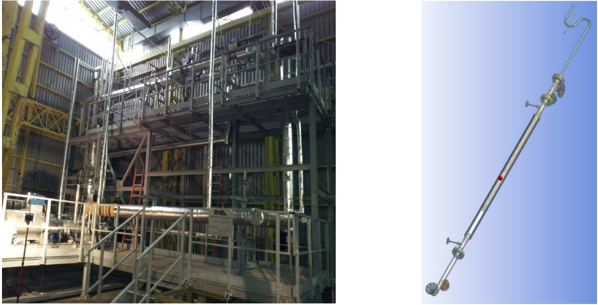
Fig. 9. View of the HELENA loop (left) and drawing of the FIV test section installed in it (right) (courtesy of ENEA).
